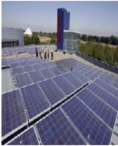
Google has installed solar panels at its headquarters in Mountain View, CA to help reduce its carbon footprint.
