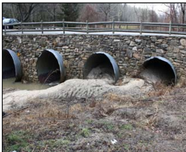
Sediment flowing into Shaw Creek from the roadside.
