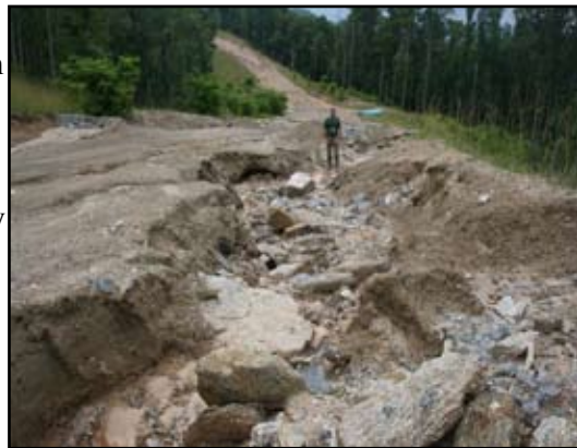
Seven Falls development deteriorating into local streams.
